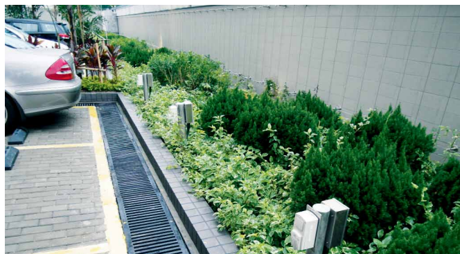
Electric vehicle charging stations in the car park
